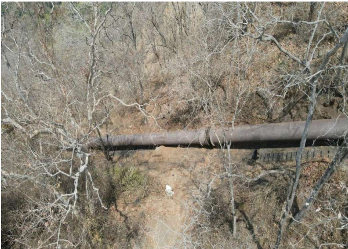
[Fig – 53] Figure showing the penstock situated in Gudalur range.
